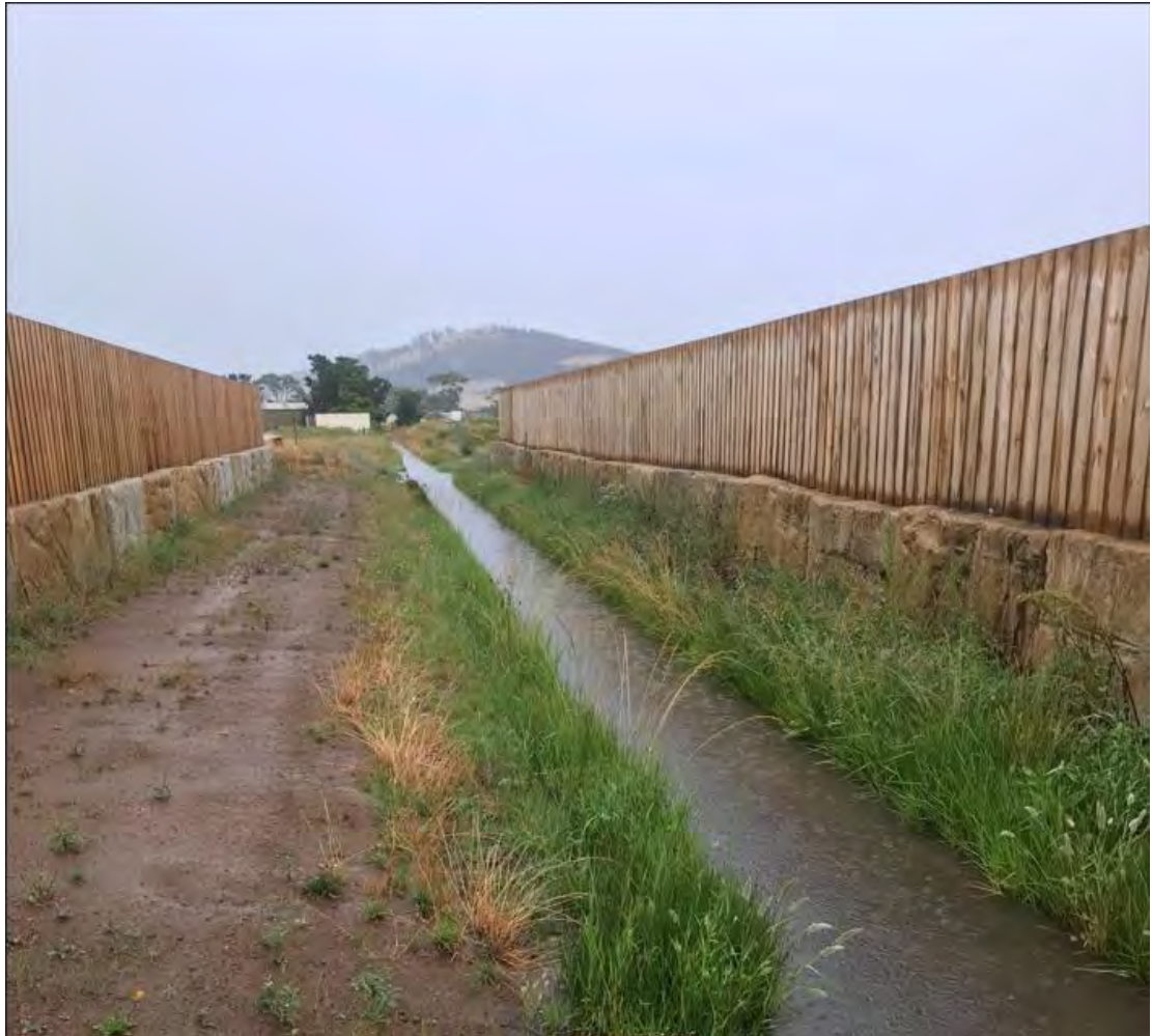
Figure 3 – Existing Sandstone stormwater channel and gravel access during rainfall event (Source: David Cundall, taken December 2021)
